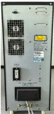
Figure 6.7.1: UPS Air Circuit Breaker on the Back
