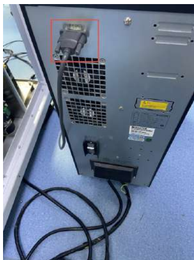
Figure 6.7.6: UPS Communication Port
